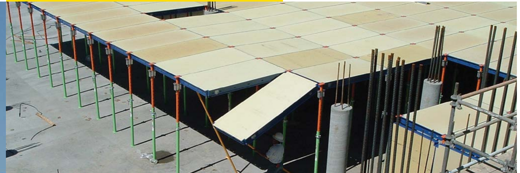
Panels, Props and ADT in use at a construction site in Washington.
